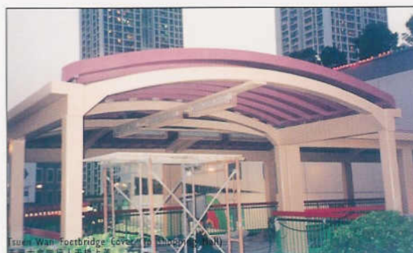
Tsuen Wan Footbridge Cover (To Shopping Mall) 荃灣大會堂行人天橋上蓋
