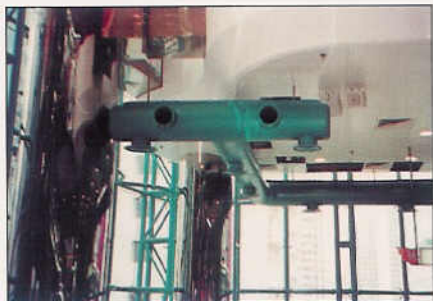
Air Duct-Tze Wan Shan Shopping Centre 慈雲山中心冷氣槽
