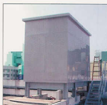
Chung On Estate Radio Equipment House 頌安邨電訊器材屋
