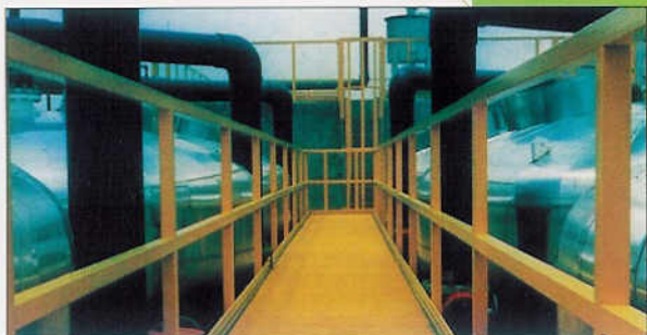
GRP Handrailing and Grating Cover
