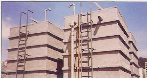
Water Tank for flusing water 咸水用儲水箱
